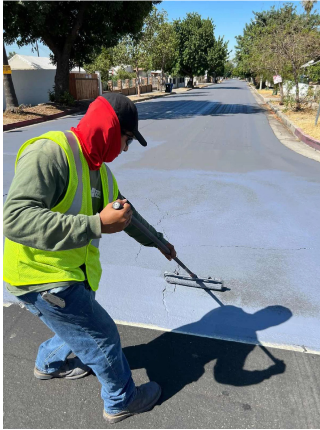
Figure 8 – A volunteer from Pacoima Beautiful applies a GAF cool coating to asphalt in the Pacoima neighborhood of Los Angeles. Source: Pacoima Beautiful.
