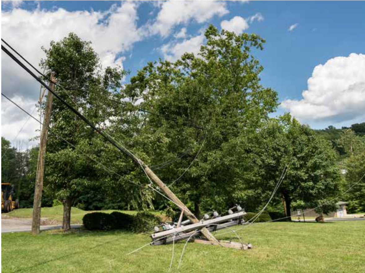
A downed power line following a storm. In the fall of 2011, nearly a quarter of a million Southern California Edison customers were without power after a windstorm toppled utility poles.
